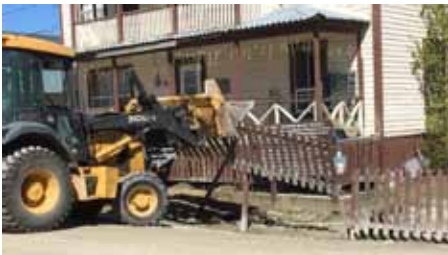
Fixing a bog hole and the foundation at Stringer House last summer. Work was also completed inside includ- ing overdue painting.
