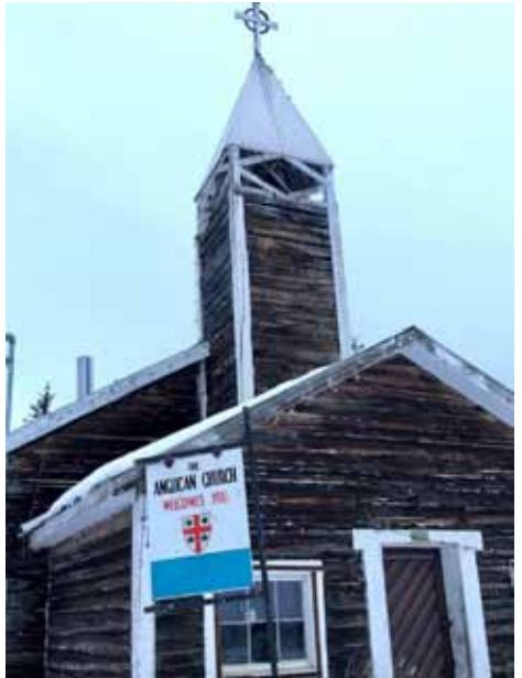
This is the "old" St Luke's, which will hopefully be repaired soon. This was built in 1959.
